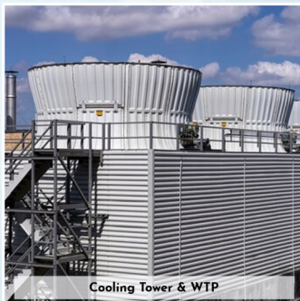
Cooling Tower & WTP
