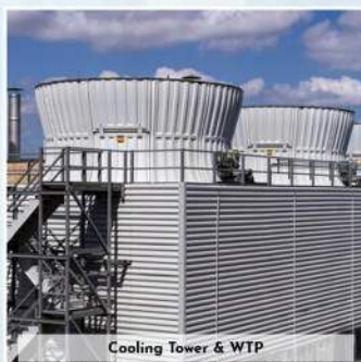
Cooling Tower & WTP
